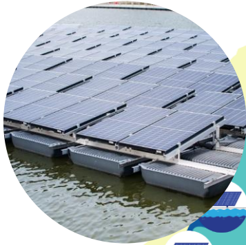
Floating Solar Modules
