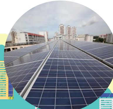
Solar Panels on Rooftops
