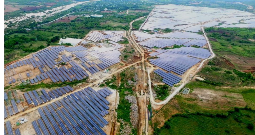
Solar Farm in Vietnam, 168 MWp
