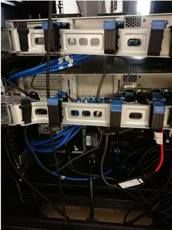
Servers and UPS
