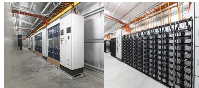
ESCRI-SA: Advanced Grid Services (Grid-forming, Virtual Inertia, 2x Fault level support) 30MW/8MWh
